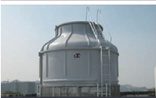
Water Cooling Tower
