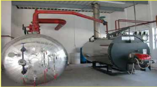
◆ Steam Boiler & Steam Accumulator
